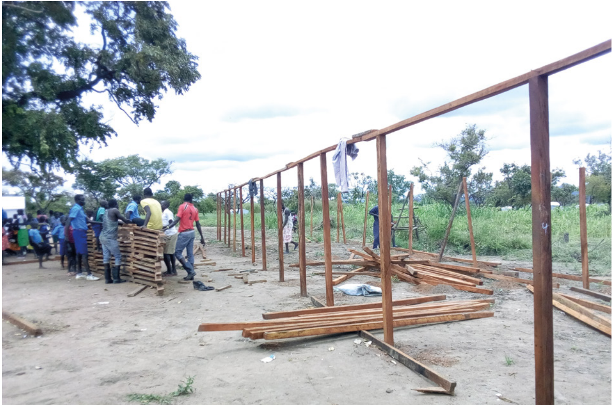
The Diocese of Liwolo lead the construction of a temporary learning space in Korijo, 2019. Photo: William Waru/Tearfund
